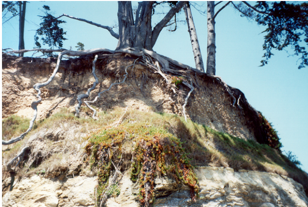
Photo 23. Exposed Cypress tree root system due to bluff erosion at 41 st Avenue.
