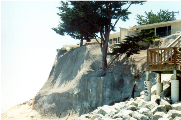
Photo 15. Private residence bluff armoring next to 41 st Avenue stairway.
