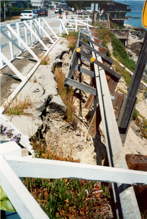
Photo 9. East Cliff Drive cliff face erosion and proposed build-out location.
