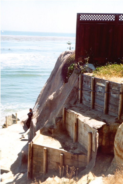
Photo 1. Private residence armoring, Adjacent to Pleasure Point Park.
