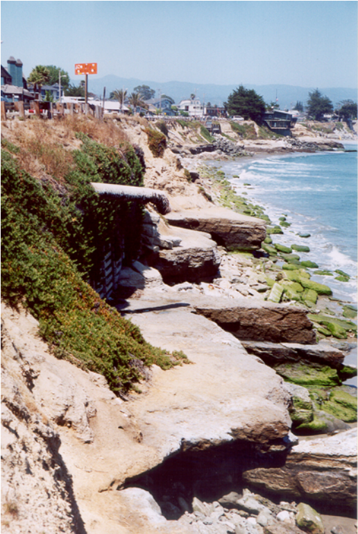
Photo 13. Wave cuts in Purisima foundation and drainage below East Cliff Drive.
