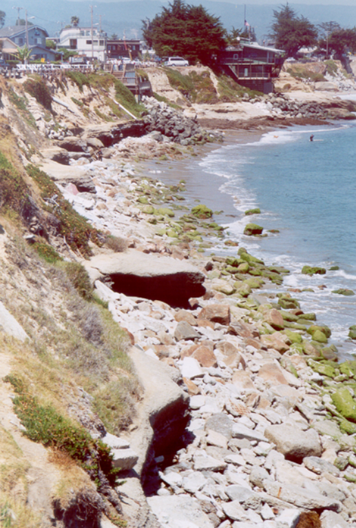
Photo 5. Rock riprap and concrete rubble, looking downcoast.
