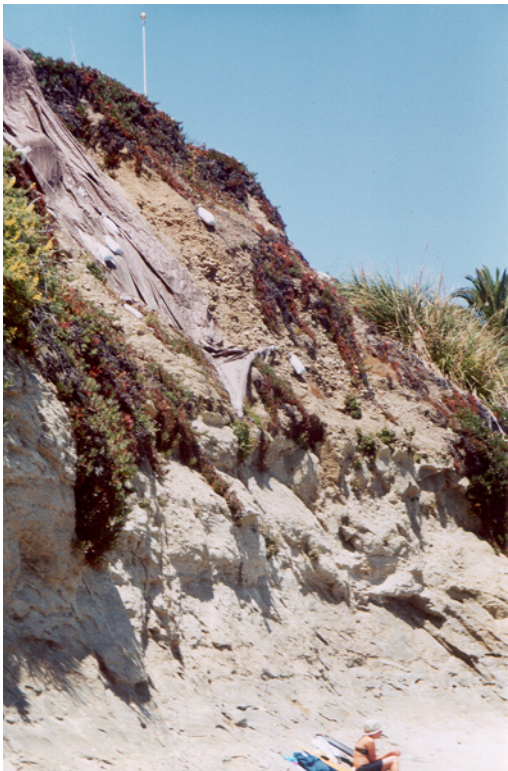
Photo 11. Erosion of the existing cliff face.
